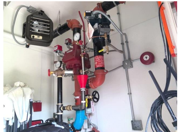
Plumbing Canes: heater not turned on.
