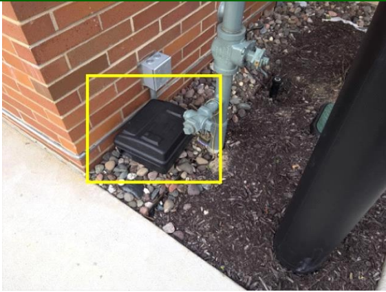
Landscaping/Rodent Traps/Exposed Wires:
