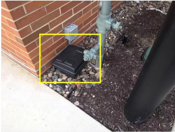
LANDSCAPING/RODENT TRAPS/EXPOSED WIRES:
