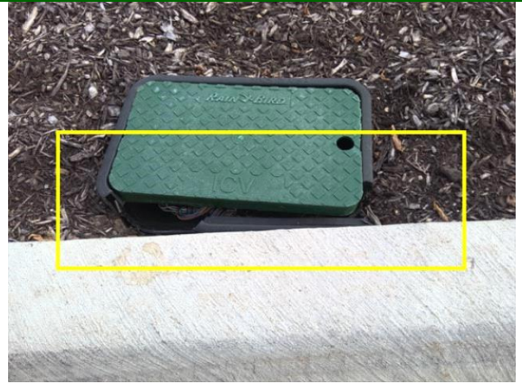
Landscaping/Rodent Traps/Exposed Wires: Exposed wires left side Raising Canes
